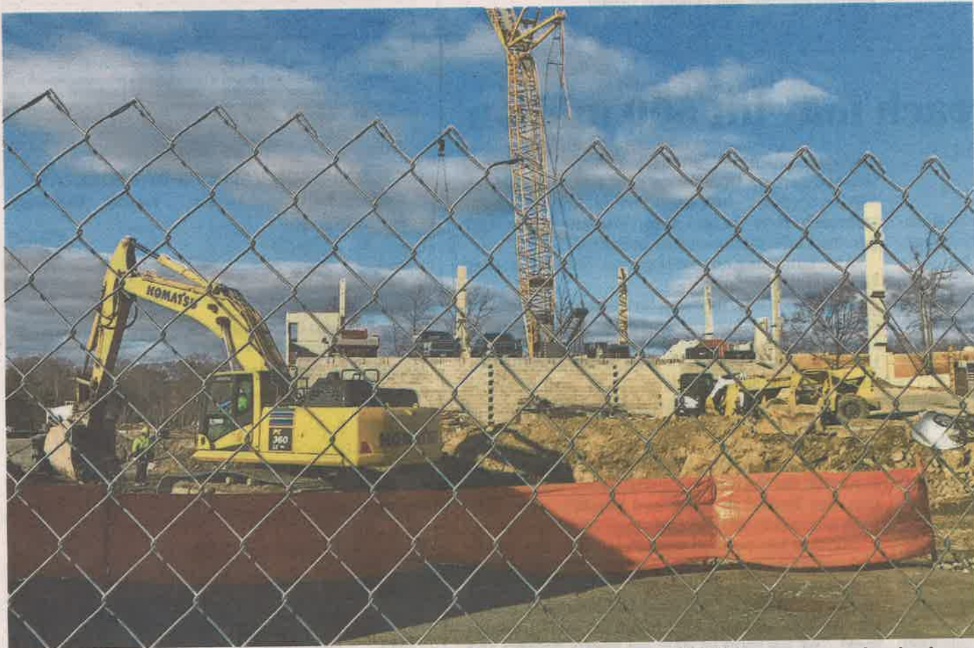
Construction of Toll Brothers' Carraway luxury apartment complex is ongoing at 103-105 Corporate Park Drive in Harrison. PHOTOS BY AKIKO MATSUDA/THE JOURNAL NEWS
